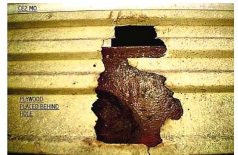
Closeup of door damage. Plywood has been placed behind the hole.
